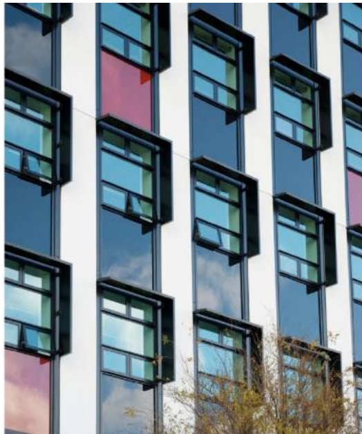
External solar shading
